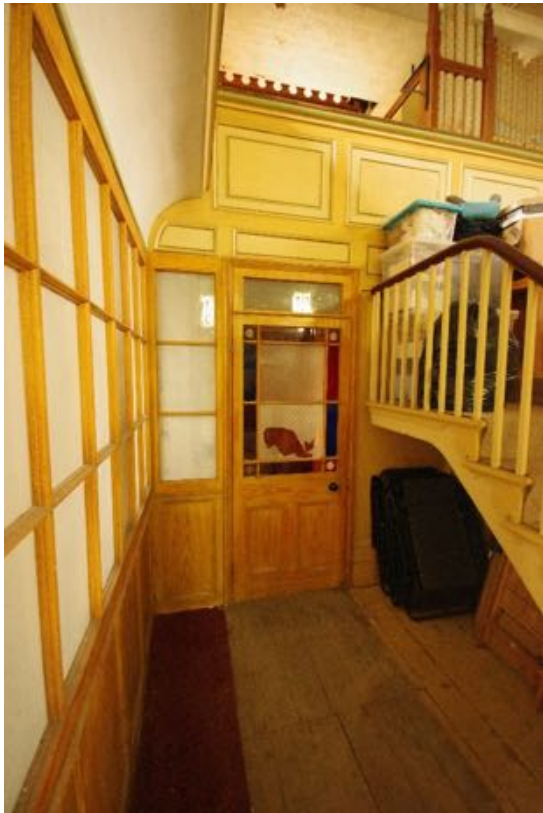
Fig 12 Glazed door with coloured glass, glazed partition to the left and balcony frontage .
