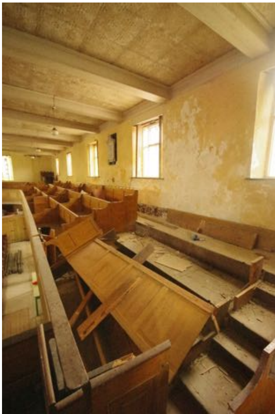
Fig 13 Damaged early 19th century box pews.
